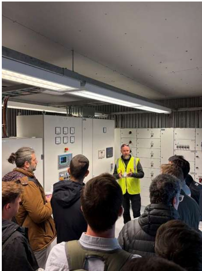
Kissakosken small hydro power plant control room visit
