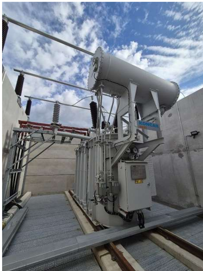
Kissakoski substation power transformer
